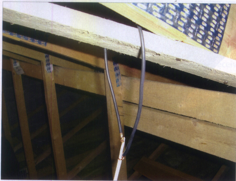
Criminal rigging This loop of co-ax was fraudulently installed as a 'high gain loft aerial'
