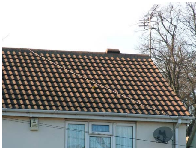
Fig 20 (left). This shot was taken from the flat roof. The diagonal cable is clipped at the top and at the bottom but not in between! This was one of a sequence of photographs taken on behalf of the Residents' Association, who were after the installer's blood!
